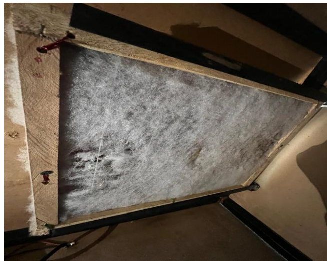
Figure 7 Wood insulated for extractor hood
